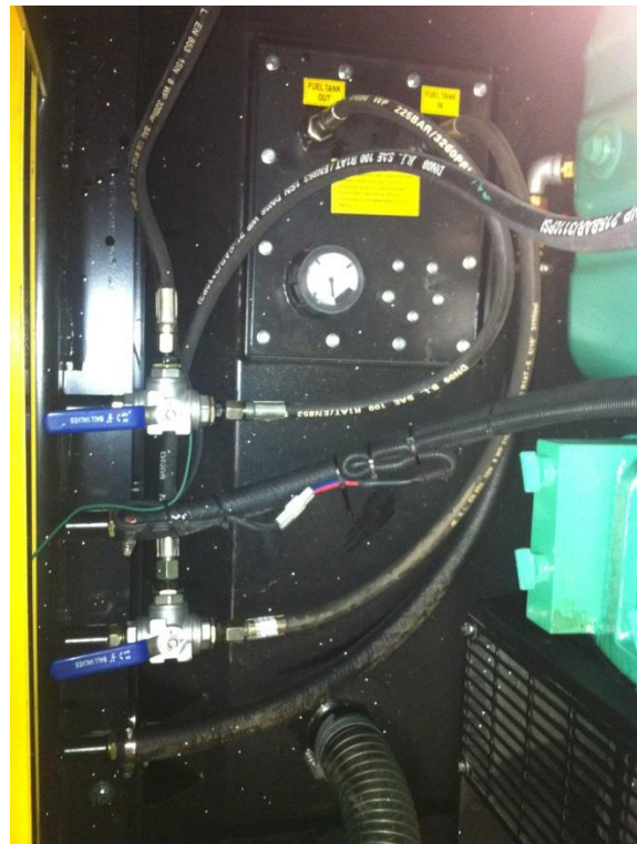
External Fuel Valves
